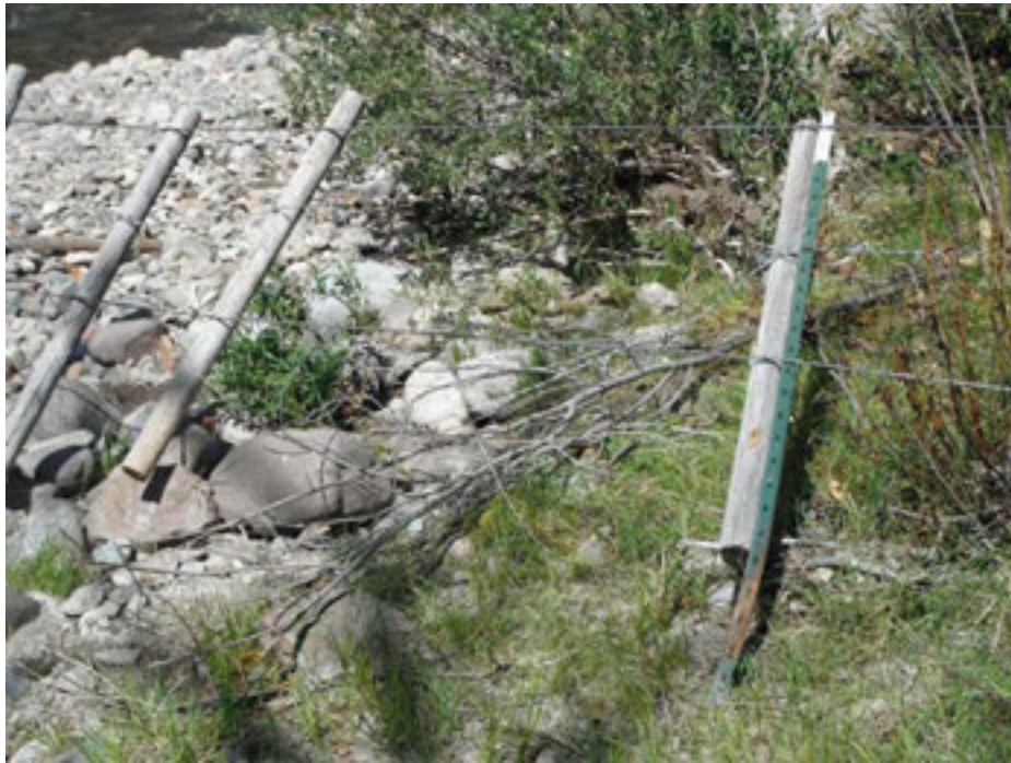
Fig. 7: West Fork ford fence, downstream side of ford, middle wire broken and posts leaning. August 11, 2012.
