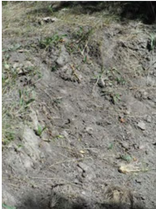
Fig. 20: Actively eroding, trampled right bank of Camas Creek, above Meyers Cove enclosure. August 2, 2012.
