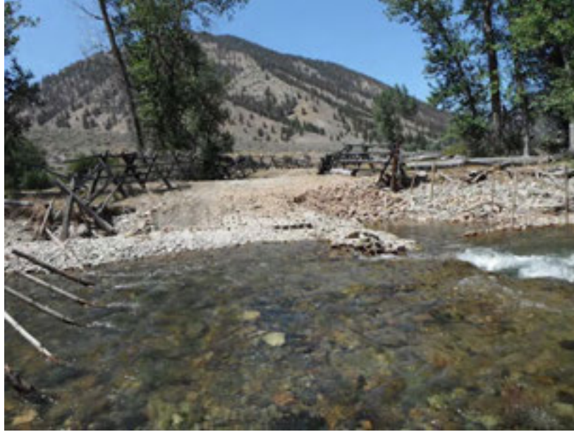
Fig. 8: West Fork ford fence, upstream side leaning precipitously. August 11, 2012.
