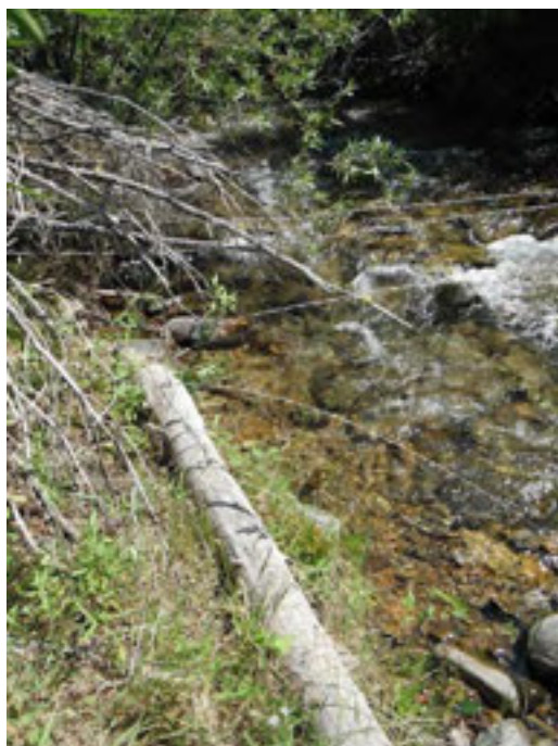
Fig. 28: Broken, loose wires on Castle Creek drift fence, across Castle Creek. August 17, 2012.
